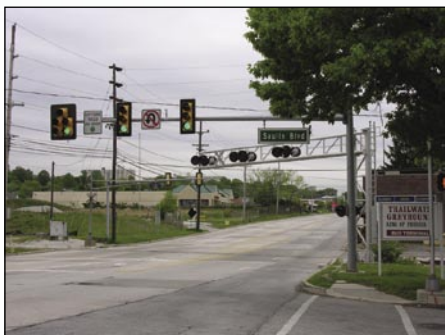
Railroad crossing signaling and traffic signals.
