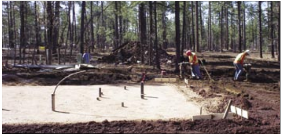
Amid the pristine trees near Pinetop, Arizona, a Henkels & McCoy crew prepares the site for one of the bathroom/shower facilities for the Hon-Dah Resort-Casino RV park.
