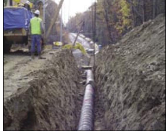
H&M Pipeline Division, replacing old 14-inch pipe with new 20-inch pipe in Pike County in Pennsylvania's Pocono Mountains for Columbia Gas Transmission. Rugged conditions warrant a double rock-shield wrap.
